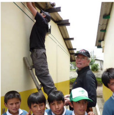
Electrical problems solved in the Colegio Viejo esp. computer lab; Paulino's Hostal, and in a classroom in Tunguiche.
